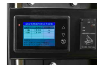
Automatic battery fire extinguishing devices
