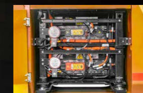
Battery and motor radiator
